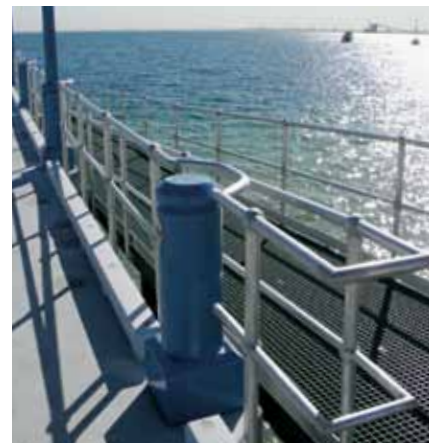
Weldlok® aluminium handrails and FRP walkway at Palm Beach Jetty, Rockingham, WA
