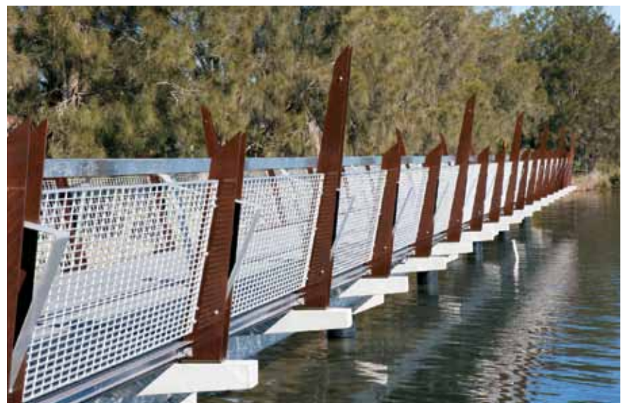
Weldlok® aluminium grating balustrades and FRP walkway at Red Bluff Shared Pathway, Lake Macquarie, NSW
